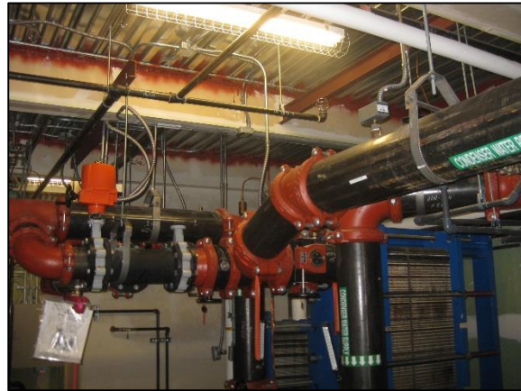
Photo A-8: Roof mechanical room—suspended piping
