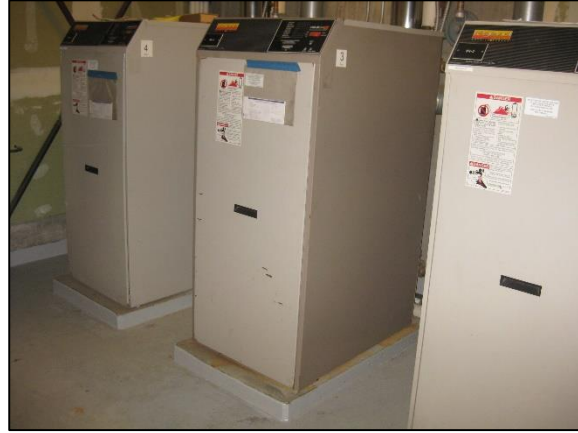
Photo A-6: Roof penthouse—boilers
