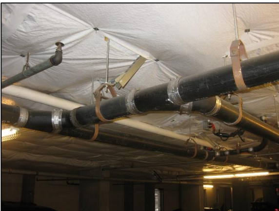
Photo A-9: Level 3—suspended drain piping
