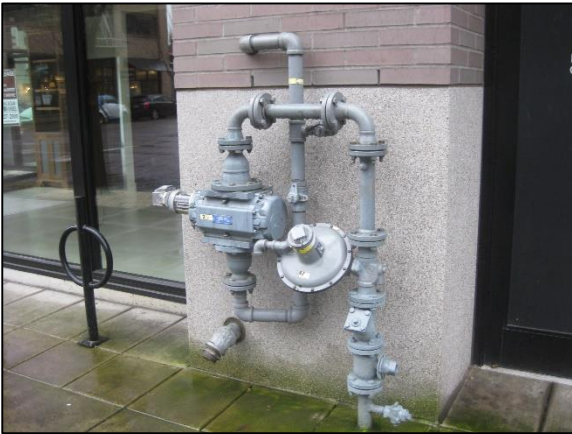
Photo A-13: Natural gas main inlet
