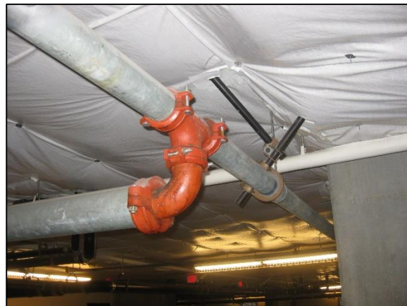
Photo A-10: Level 3—suspended sprinkler piping
