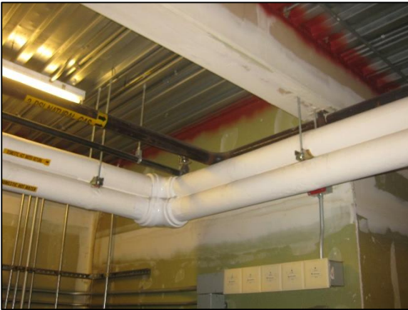
Photo A-7: Roof penthouse—suspended piping
